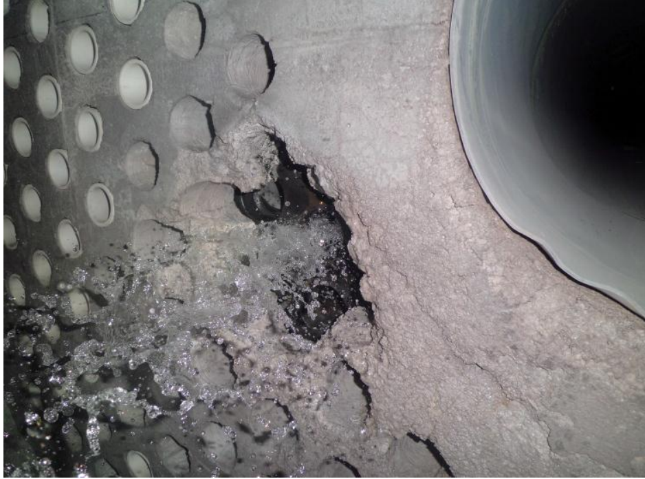
Figure 2: Heavy water leakage was observed at the inlet tube sheet
