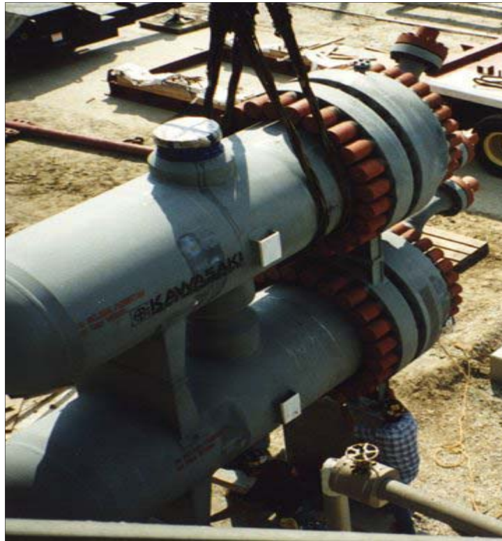
FIGURE-3: Ammonia Converter exit waste heat boiler
