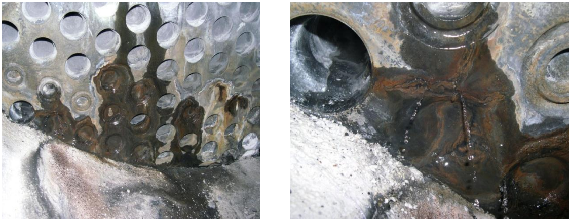
Figure 9 and 10: Cracks in outlet tube sheet
