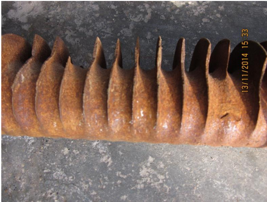
Figure 1: severe acid corrosion of economizer tube
