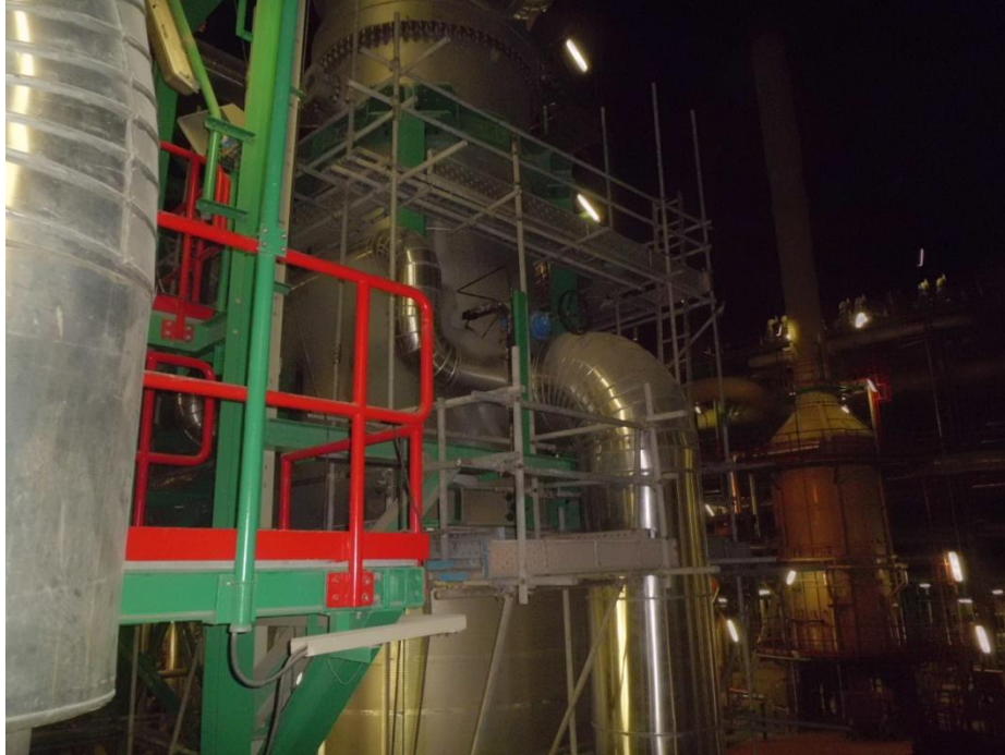
Figure 1: Leaking Process gas bypass valve of E0309
