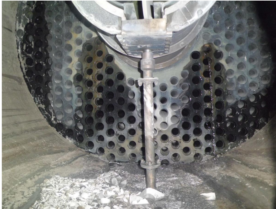
Figure 4: Water and debris was found at the outlet compartment
