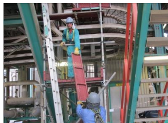
Wrong Method (standing under hanging load)
